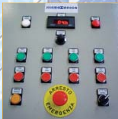
PARTICULARITES PANNEAU DE CONTROLE PARTICULAR PANEL DE CONTROL
